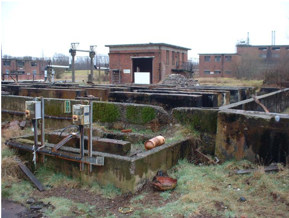
Plate 6.2 - Acid tank farm (22/102H). Concrete supports show signs of acid erosion.
